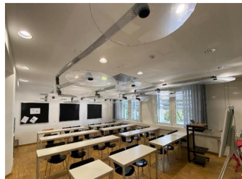
Figure 1: MPIC-MEV system installed in a TU Graz lecture room
