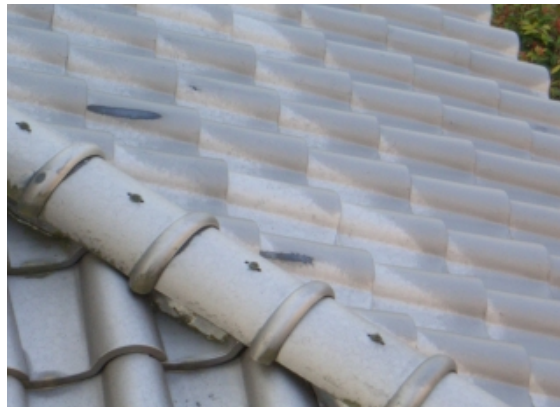
Figure 2 Surface Condensation on roof tile
