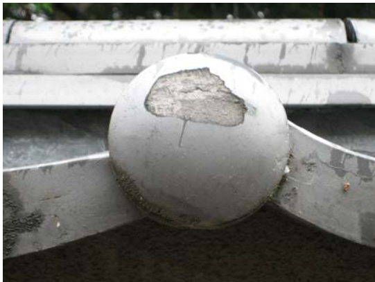
Figure 1 Roof tile damaged by freezing (Kyoto)
